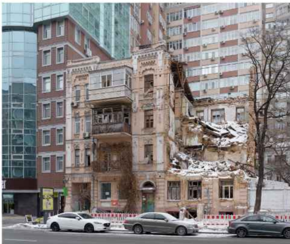
The building after the shelling, front view, 2020
