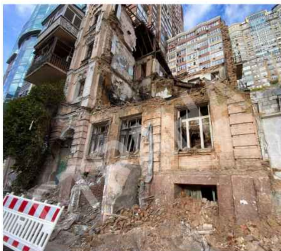
The building after the shelling, lower part of the building, 2021
