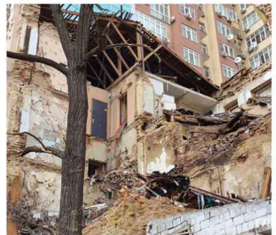
The building after the shelling, upper part of the building, 2021
